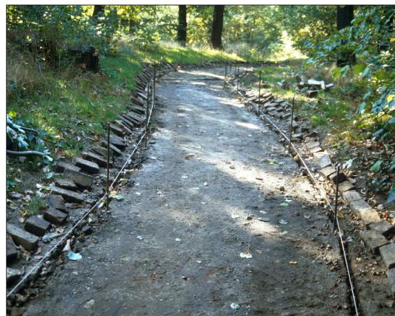
figure 3: Restoration of a historic footpath in Babelsberg Park near Potsdam. The picture shows the curved line direction which is marked by iron nails and white bands during adjustment of the interlayer's surface. All material like the recovered original edges of 'Bernburger lime stone' were recorded, photographically documented and were part of a comparative investigation with historic landscape construction theory in relevant manuals. photo: TU Berlin, October 2001.
